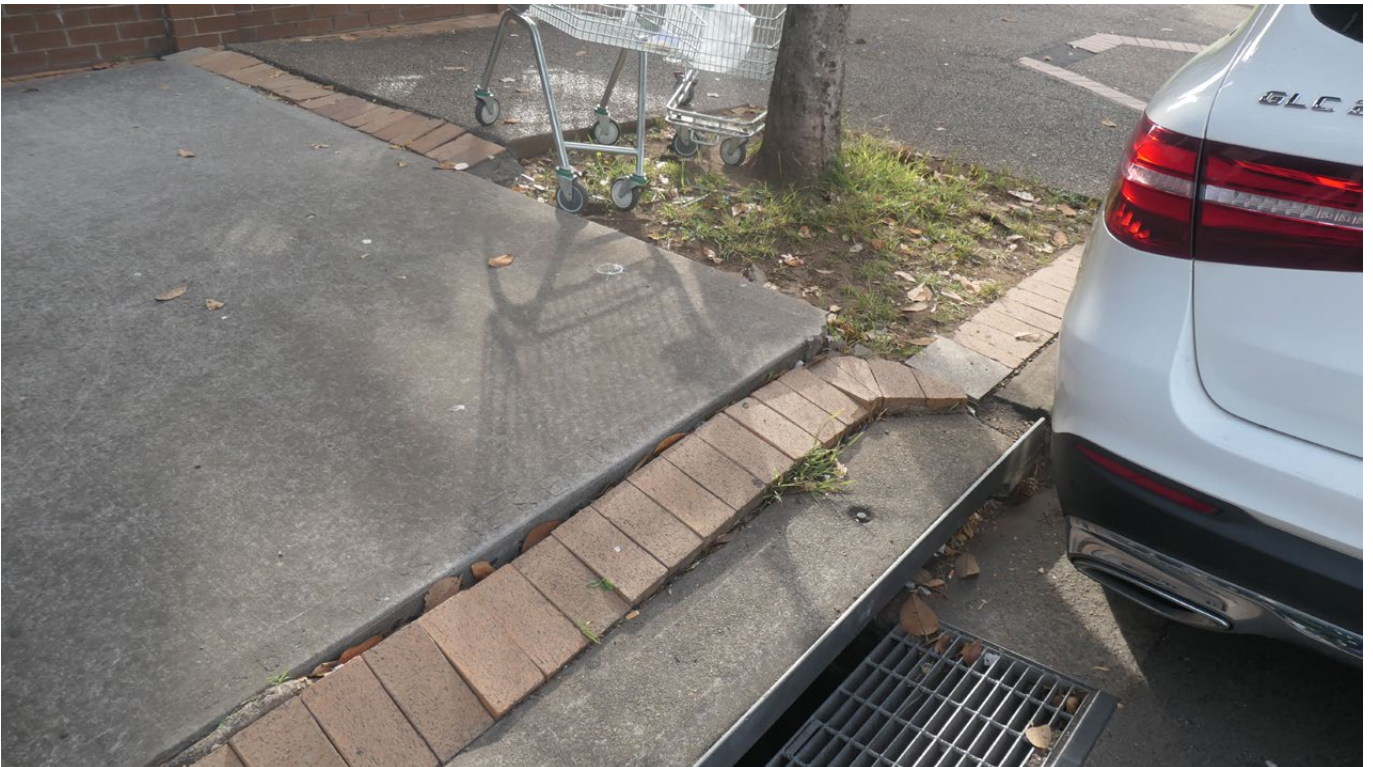
Figure 11: Insufficient preparation of planting areas and lack of the provision of soil volume for adequate tree growth is one of the leading causes of longer term costs and liabilities for the community and should be better addressed as part of Council's Tree Management Strategy and guidelines moving forward to help minimise longer term issues and liabilities. (Source: Arterra)
