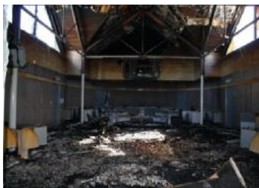
Fire damage to Council's administration centre on Hoxton Park Road
