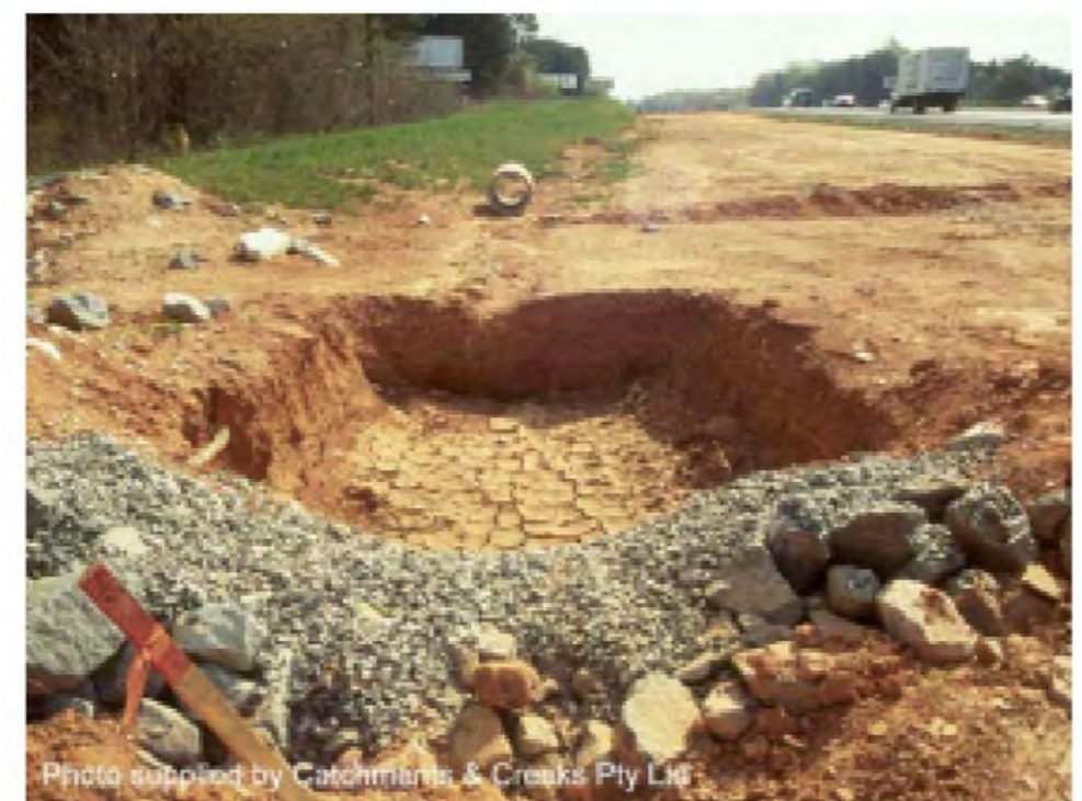
INTERIM SILT TRAP
