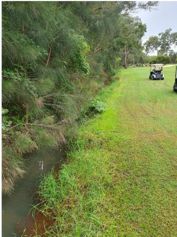
Figure 7 - Indicates the initial west - east section of the Stage 2 development. The current drainage channel is to be infilled for the pathway and a new channel trenched in a location parallel to the current about 3m to its south. The trenched material will be used to infill the current drainage channel
