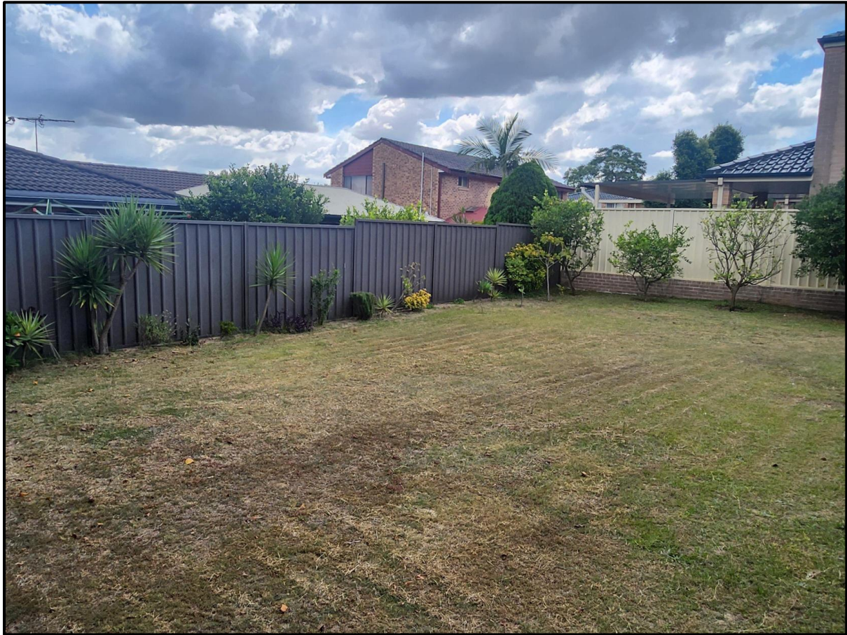
Figure 4: Northwest corner showing northern fence sitting atop retaining wall where the proposed 4m tall acoustic fence is proposed.
