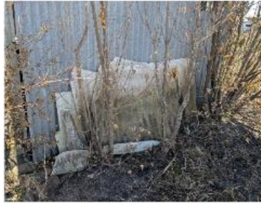
1. External, south east shed 3, redundant panels to rear of shed - fibre cement sheet
