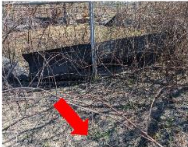
3. External, east of horse yard, spalling debris - fibre cement sheet
