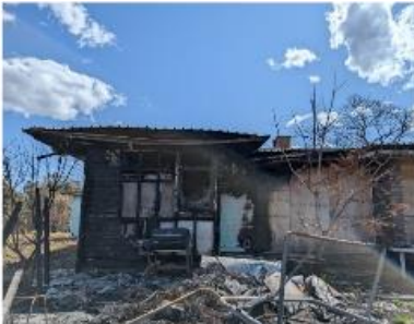
9. Fire damage to east side of house.
