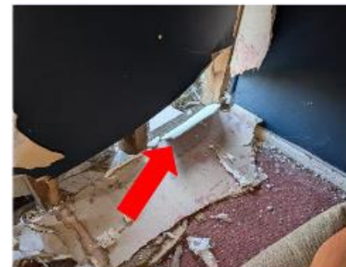
12. Minor asbestos contamination within the bathroom of the house via a pre-existing penetration in the wall.
