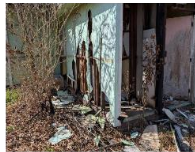
5. Significant damage to fibre cement wall linings by vandals.
