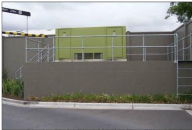
Figure 51 - Example substation raised above 1:100 flood level
